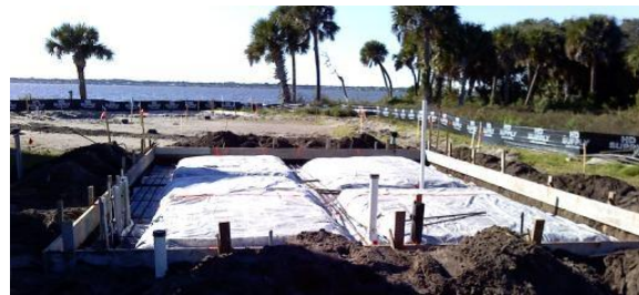
Figure 2. Site work underway prior to pouring concrete pad for broodstock tanks at CPL.
